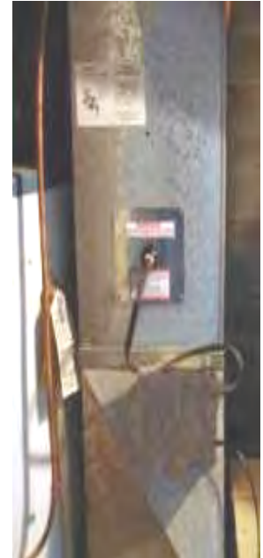
Installed UV tube in Air Duct
