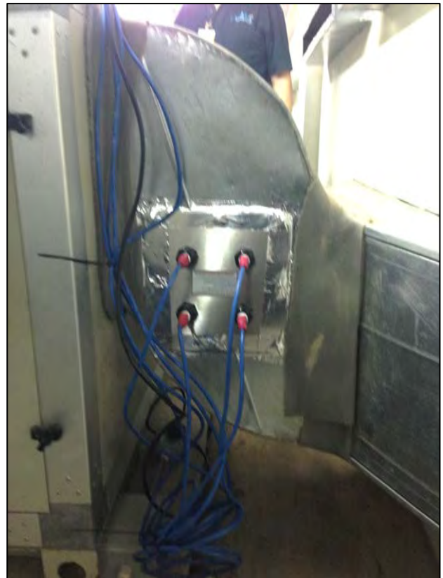
Right side of theatre 4 UV tube installation
