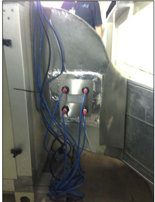
Right side of theatre 4 UV tube installation
