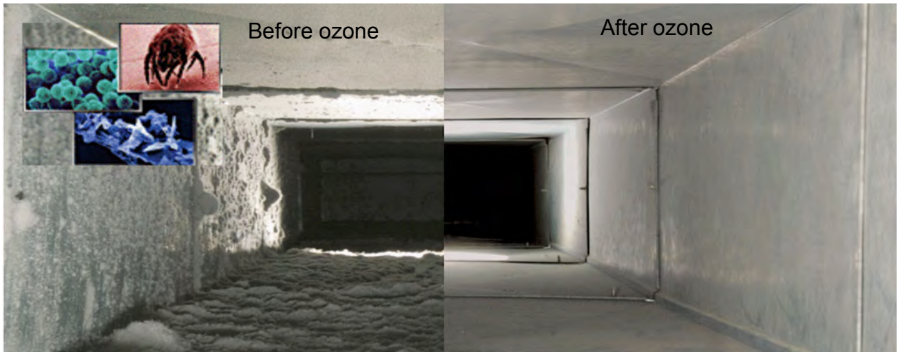
Typical kitchen or commercial building exhaust duct
