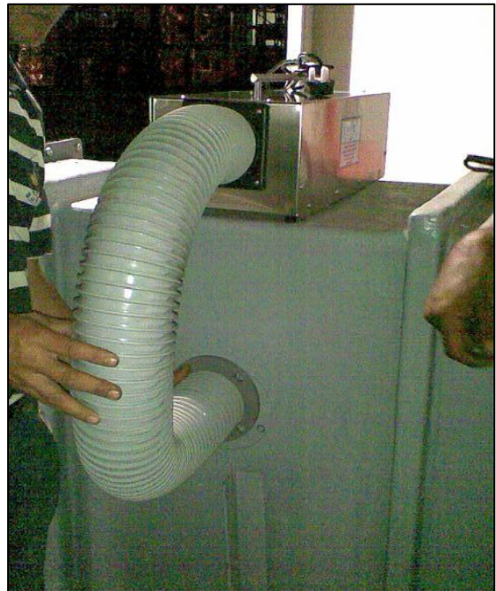
ProMedUSA UV SG7000 PRO Ozone Generator installation
