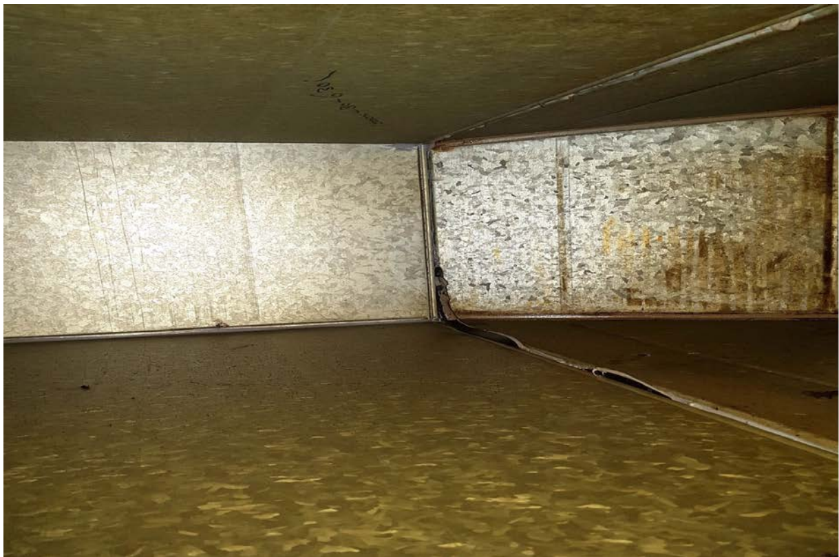
After installation of ProMedUSA Duct Ozone System
