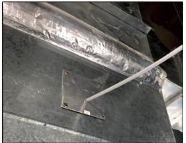
Ozone In-Duct Insertion
