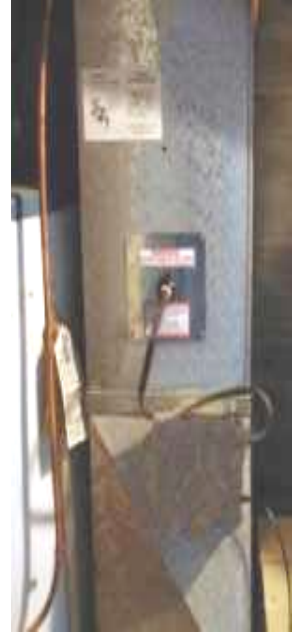
Installed UV tube in Air Duct
