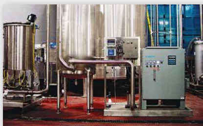
CD6000HO - Food Processing Facility
